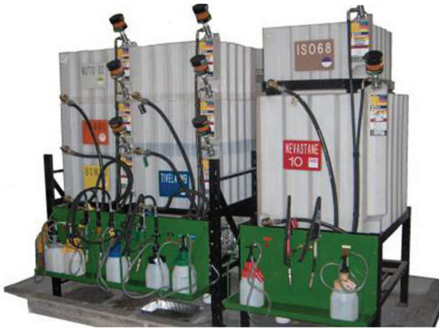
Figure 6. Custom lube tank dispensing stand. Oil is filtered going in and coming out.
