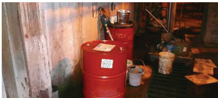
Figure 11. A service call reveals multiple sources of oil contamination.
