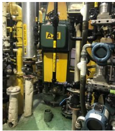
Indoor mixing gearboxes
