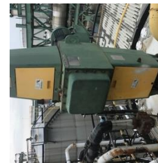
Outdoor mixing gearboxes
